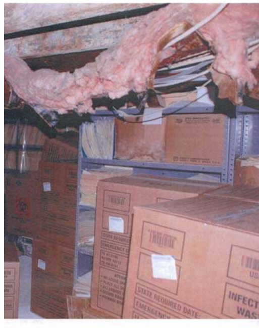
Boxes of bio-hazardous waste in basement
